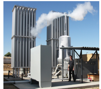
LN2 and LH2 pumping and vaporization station
