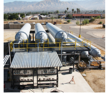
5,000 ft 3 of total facility gas storage at 5,500 psi
