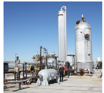
Steam test pad with high pressure steam vessels
